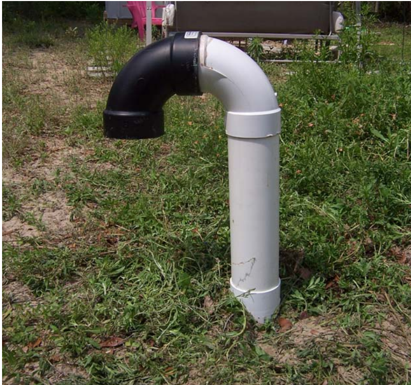
Figure 16. Picture taken on 04/14/09 of a vent pipe typical of FAST installations. Note the PVC coupling at ground level. In order to take a sample, the pipe was cut and repaired with the coupling. The black piece is a charcoal filter installed due to odor complaints. In this neighborhood, there are 5 systems in a row, backing to another 5 systems. This resulted in 10 systems on 1 ¼ acre which apparently created an odor problem.
