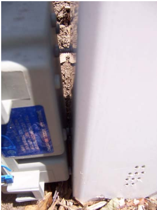
Figure 13. Picture taken on 04/16/09 of Norweco system with the wiring to the control box not connected. There was power to the pump, but not to the aerator control box.
