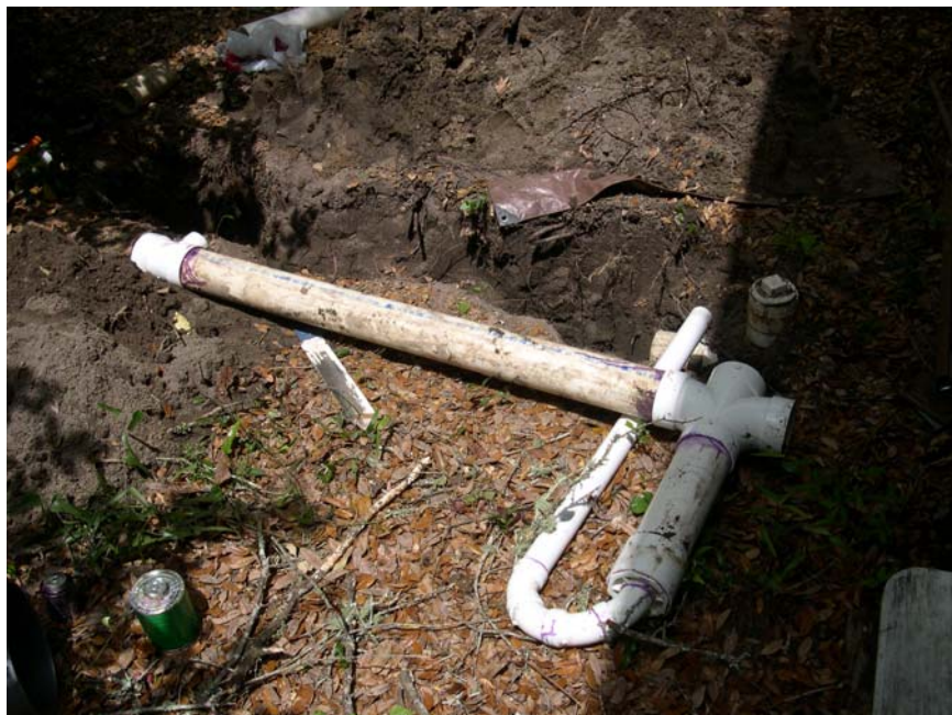
Figure 7. Plumbing for sampling raw wastewater about to be installed between the house and septic tank at site WSS-4-2. The water sensor is placed in the 4 inch opening of the 4-way PVC piece. Note the inlet clean out.
