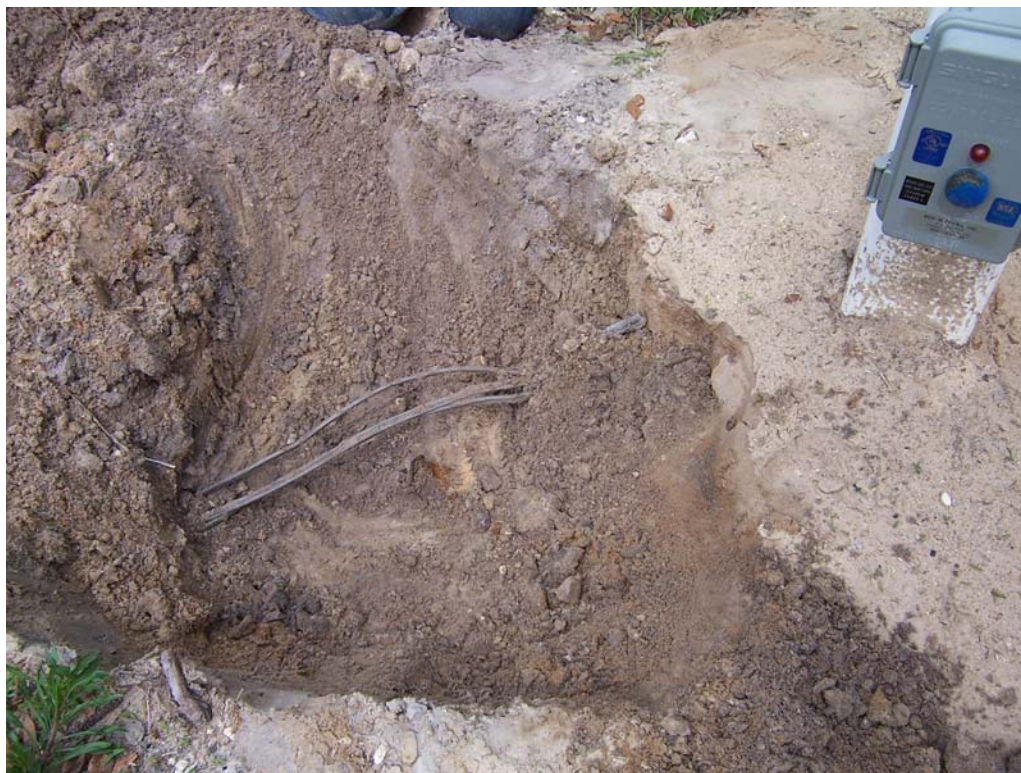
Figure 15. Picture taken on 04/20/09 of Norweco system with wires strung across the pump tank lid preventing access. No sampling port was installed. Maintenance records indicate the effluent was visually inspected.
