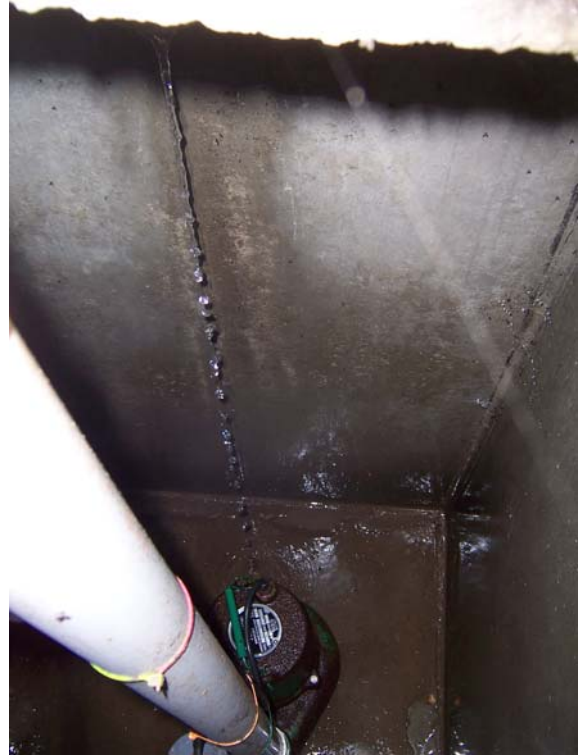
Figure 14. Pictures of the inside of an empty pump tank attached to a functioning FAST system. The installer indicated that a plug at the bottom of the tank came out and has encountered this problem at other sites.
