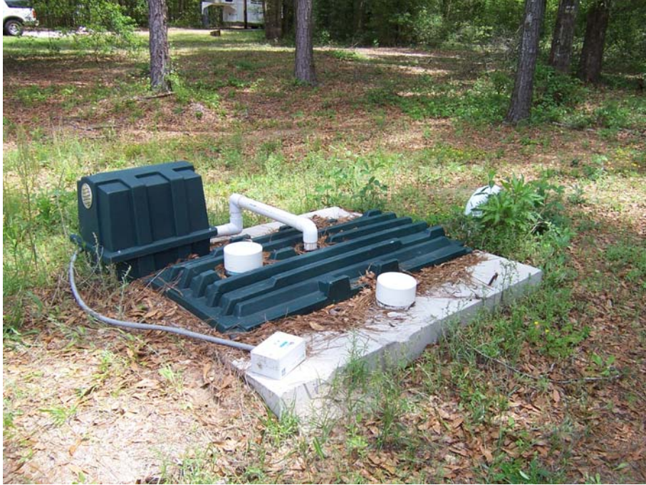
Figure 12. Picture taken on 04/16/09 of a FAST system with the unwired control box lying on the exposed tank. The system was in use with sewage, but no electricity.
